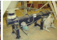
Installed Electromechanical Tube Feeder
